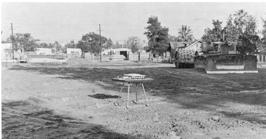
BELOW —Scale model stands alone in middle of Dining Hall building site.
